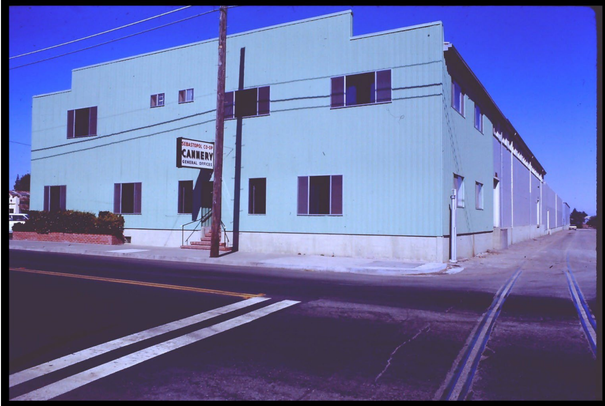
Figure 14 This 1970 photograph shows that original, circa 1924, fenestration and siding of the façade and side elevations of 6782 Sebastopol Avenue had been replaced with manufactured wood siding, known as T1-11 and fixed and sliding aluminum frame windows. Note that a contemporary sign of backlit plastic sign above the entrance reads “Sebastopol Co-op Cannery.” (Courtesy of the online photographic archives collections of the Western Sonoma County Historical Society, accessed via the Sonoma County Library).
