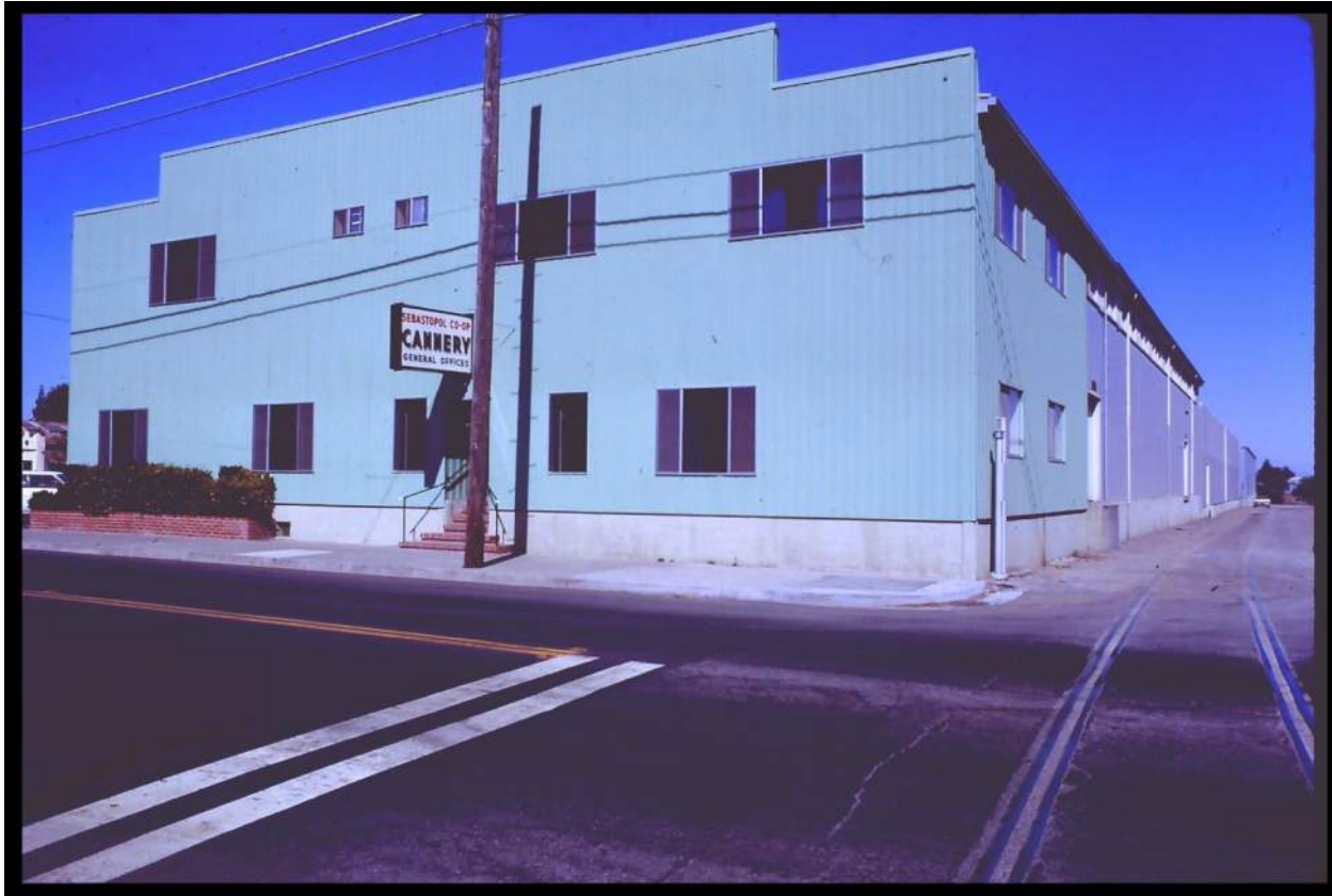
Figure 15 This 1970 photograph shows that original, circa 1924, fenestration and siding of the façade and side elevations of 6780 Sebastopol Avenue had been replaced with manufactured wood siding, known as T1-11 and fixed and sliding aluminum frame windows. Note that a contemporary sign of backlit plastic sign above the entrance reads "Sebastopol Co-op Cannery." (Courtesy of the online photographic archives collections of the Western Sonoma County Historical Society, accessed via the Sonoma County Library).
