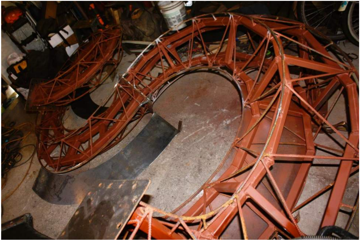
Here is a photo of the internal structure of one of my sculptures. This is before I add the corten steel sheeting. You can see one of the panels in the middle left of the photo before it is welded on.
