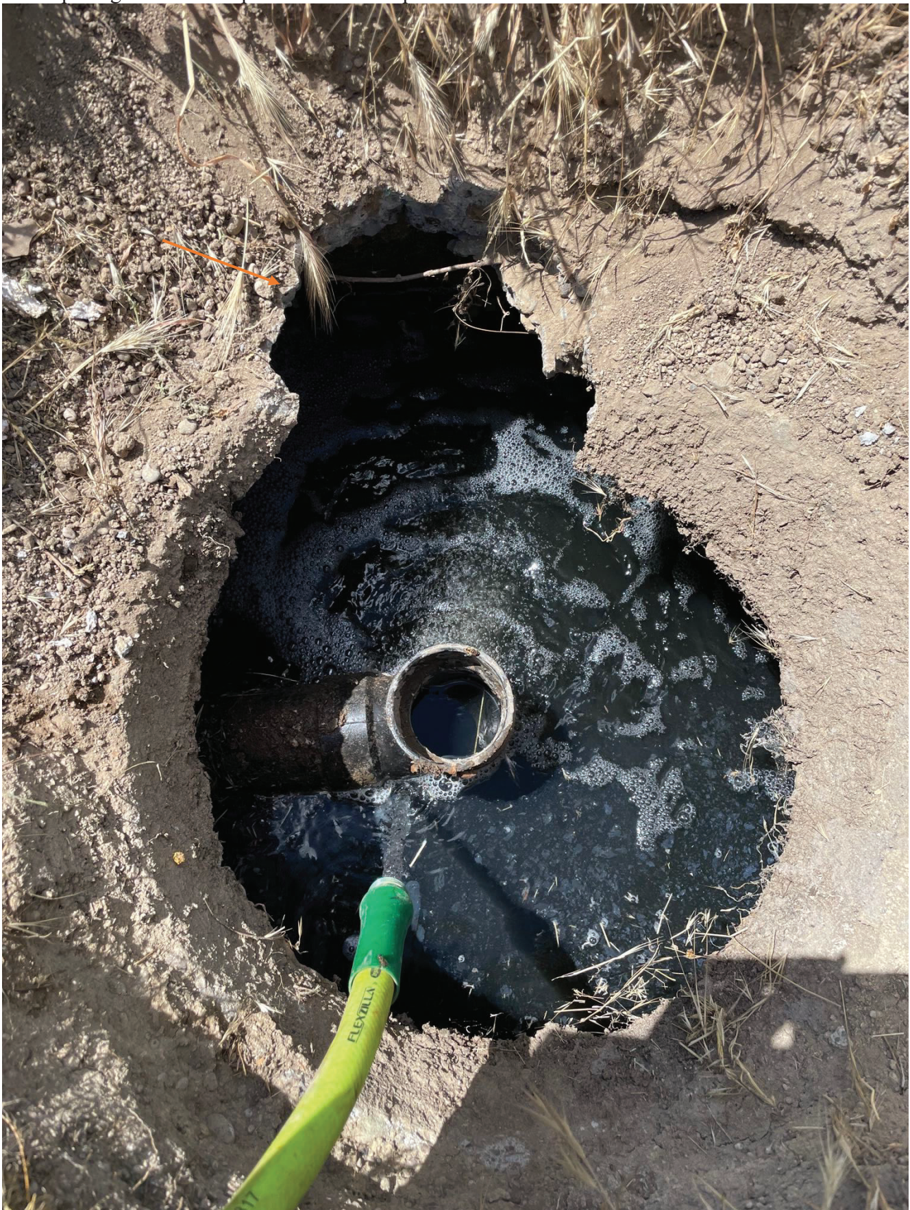
Hole/opening at outlet compartment of the Septic Tank
