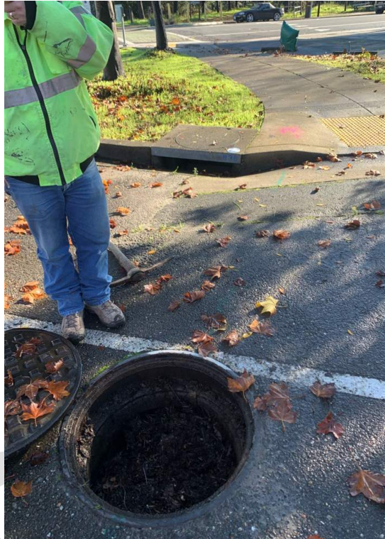
Figure 5 GHD staff at a manhole upstream from Petaluma Ave. with sediment accumulation at the manhole rim along the southern run of Reach 3 along a run of 6'x3' arched concrete conduit.
