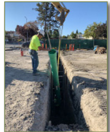
Bella Creek Apartment Complex: Underground Utility Installation for New Seven Building, 92-Unit Residential Community.
